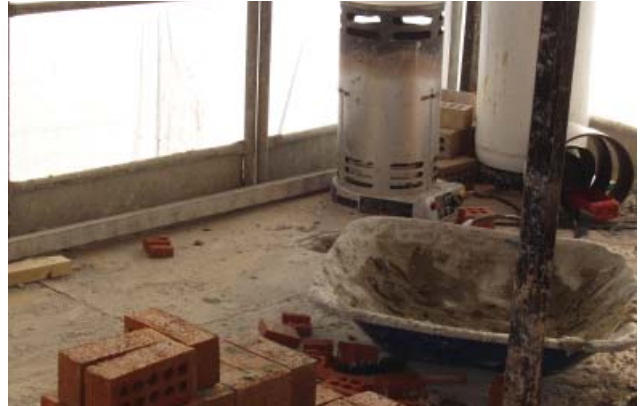
Photo 5 Space Heater in Enclosure
